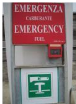
EMERGENCY FUEL STOP BUTTON LOCATION
